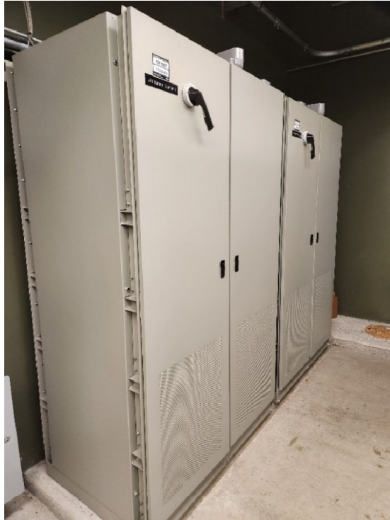
Figure 18: Photo 5 Battery Cabinets
