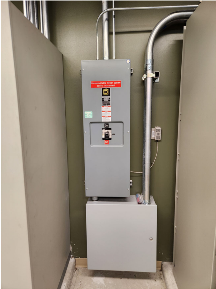
Figure 5: Wall Mounted Battery Disconnect (UPS to the left and Battery Cabinets to the right of the Battery Disconnect)
