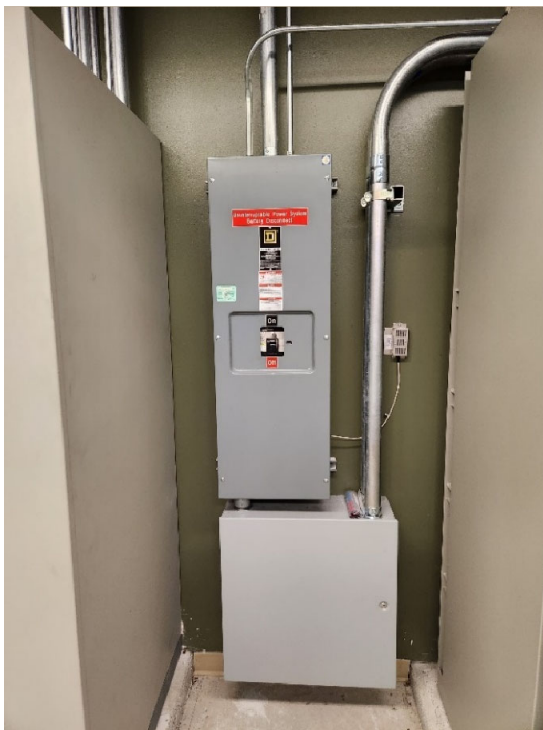
Figure 17: Photo 4 Battery Disconnect
