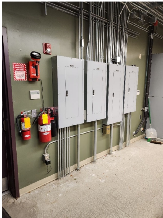
Figure 21: Photo 8 Electrical Distribution Panels
