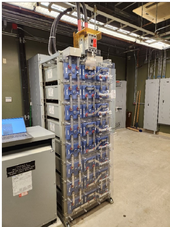
Figure 27: Transformer DB and DC Rectifier Batteries
