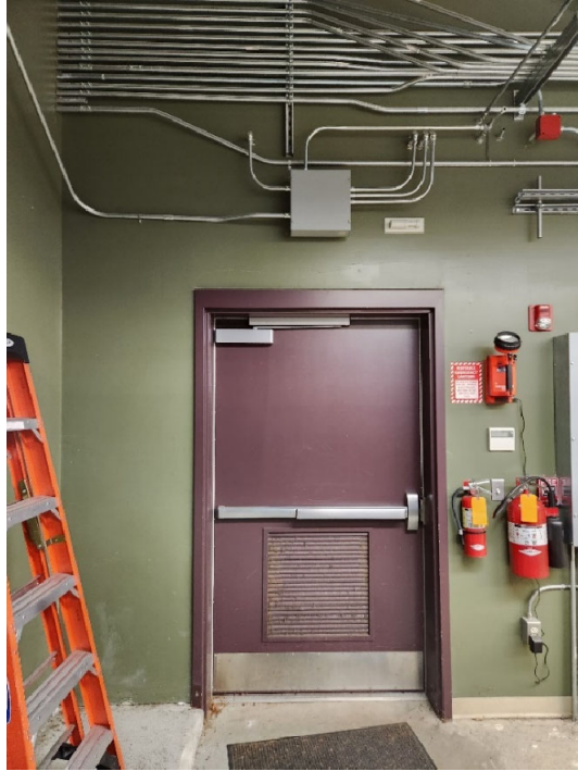
Figure 20: Photo 7 Exterior Electrical Room Door (48 inch to ground level, no curbs)
