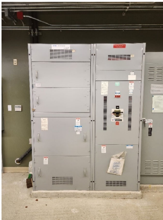
Figure 23: Photo 10 Utility Power Main Disconnect and Current Transformers (Front View)
