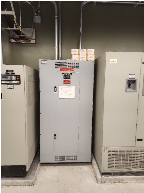
Figure 15: Photo 2 Maintenance Bypass Cabinet
