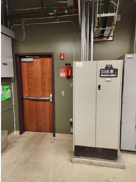
Figure 14: Photo 1 Electrical Room Interior Door and PDA
