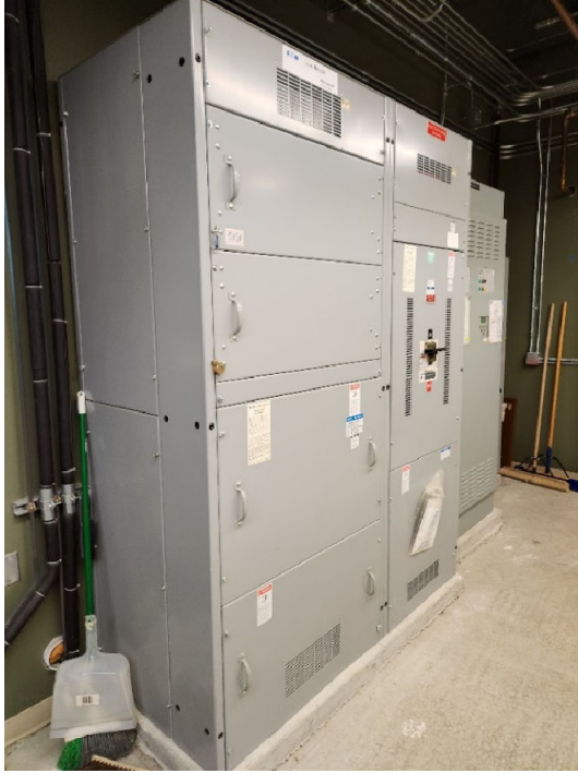
Figure 22: Photo 9 Utility Power Main Disconnect and Current Transformers
