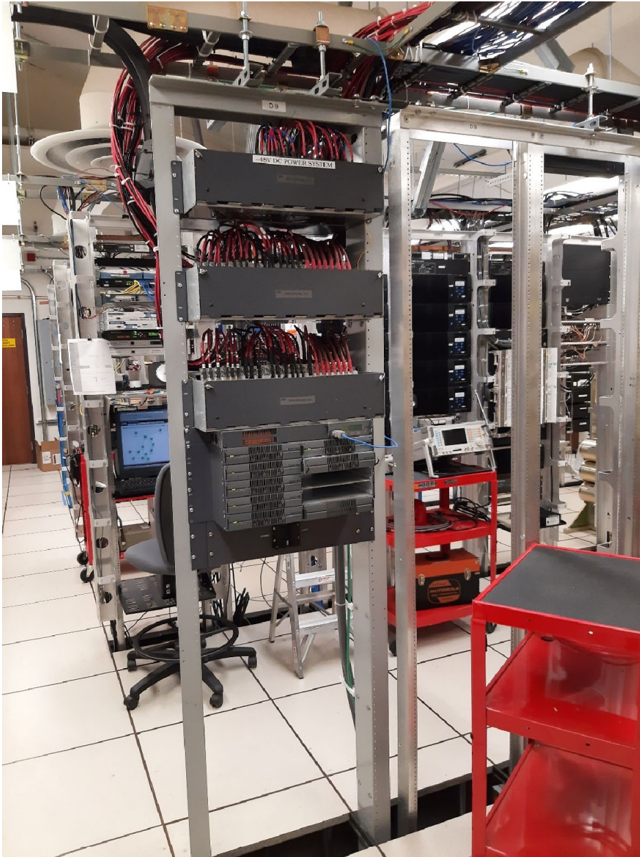
Figure 1: 911 Carver St. (Cencom) DC Power Rack
