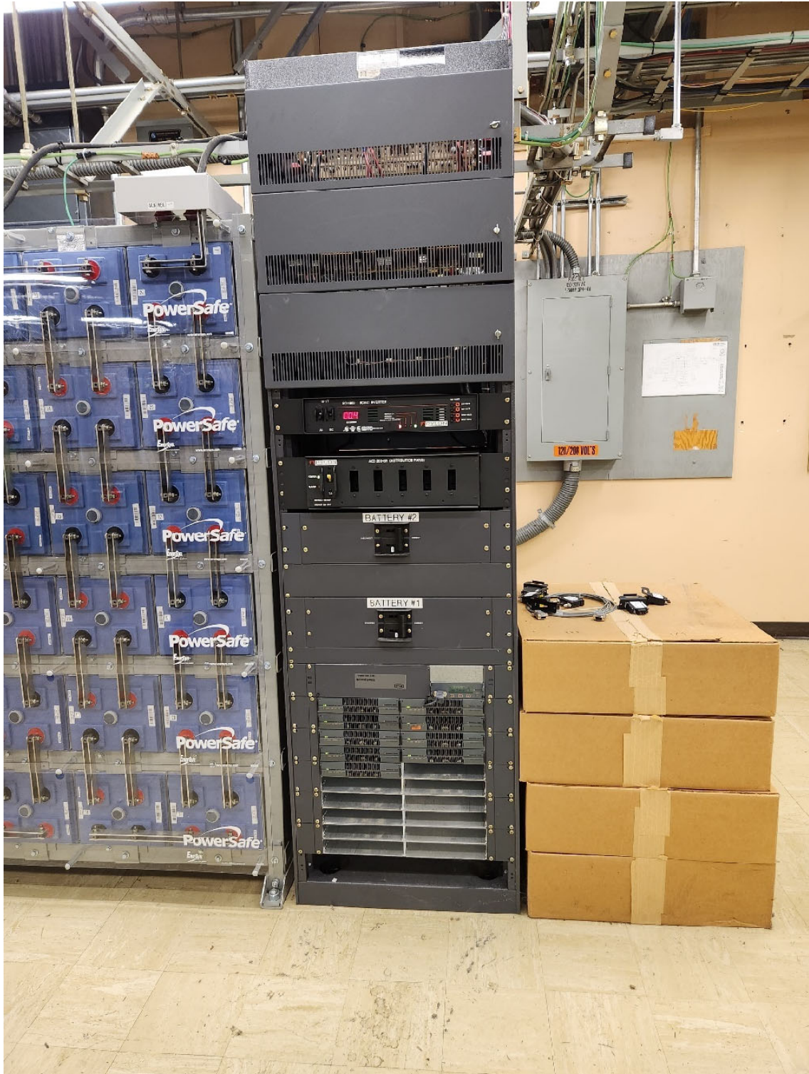
Figure 6: Gold Mountain DC Power Cabinet
