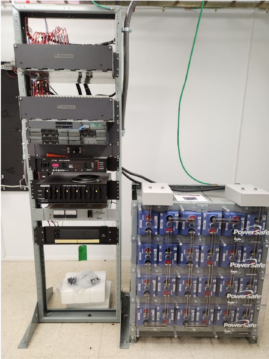
Figure 18: Purdy DC Power Rack and Battery System
