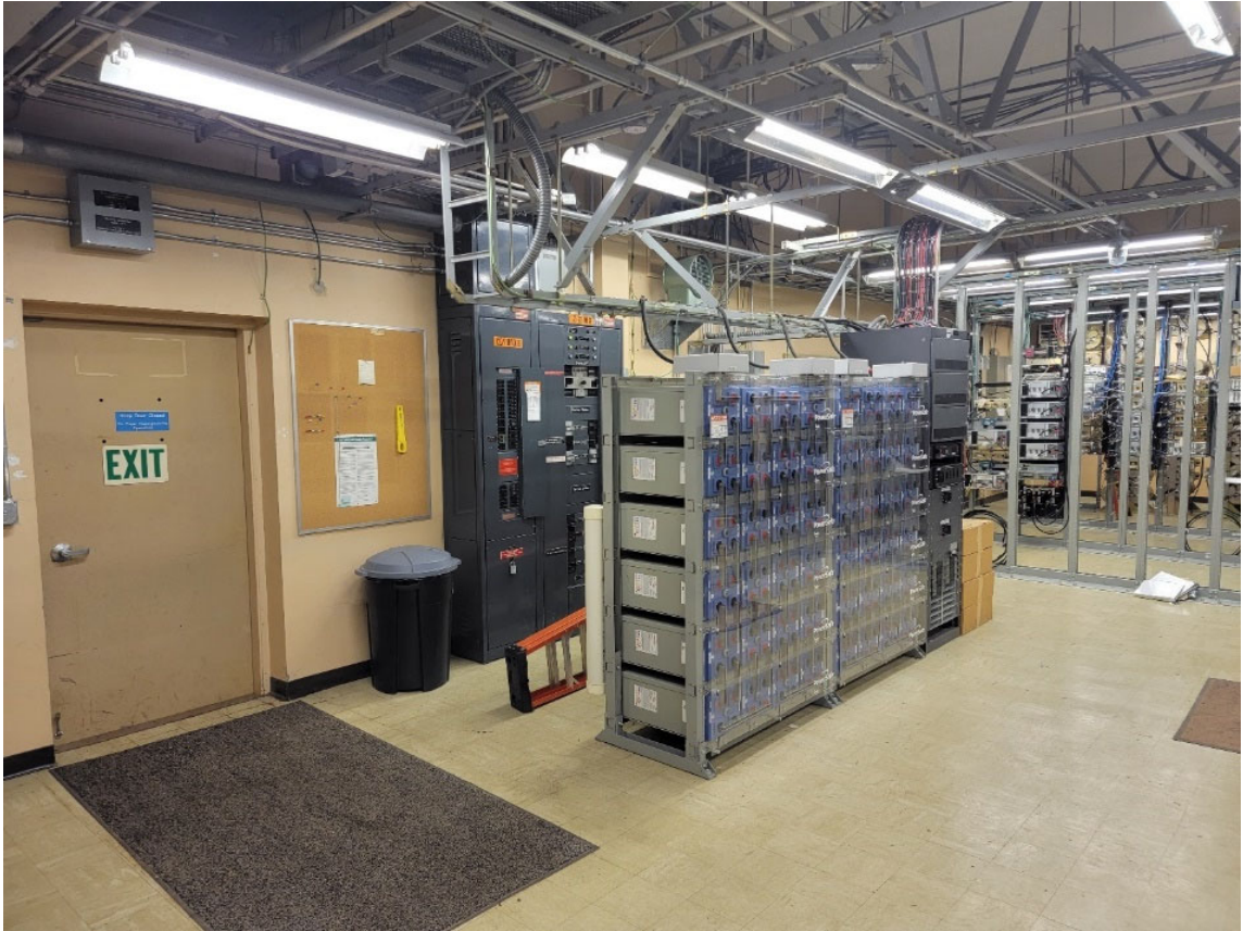
Figure 5: Gold Mountain Batteries and DC Power Cabinet
