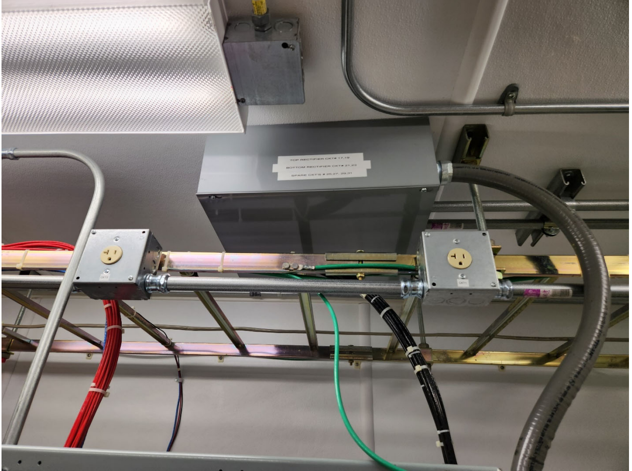
Figure 19: Purdy Site AC Power Junction Box
