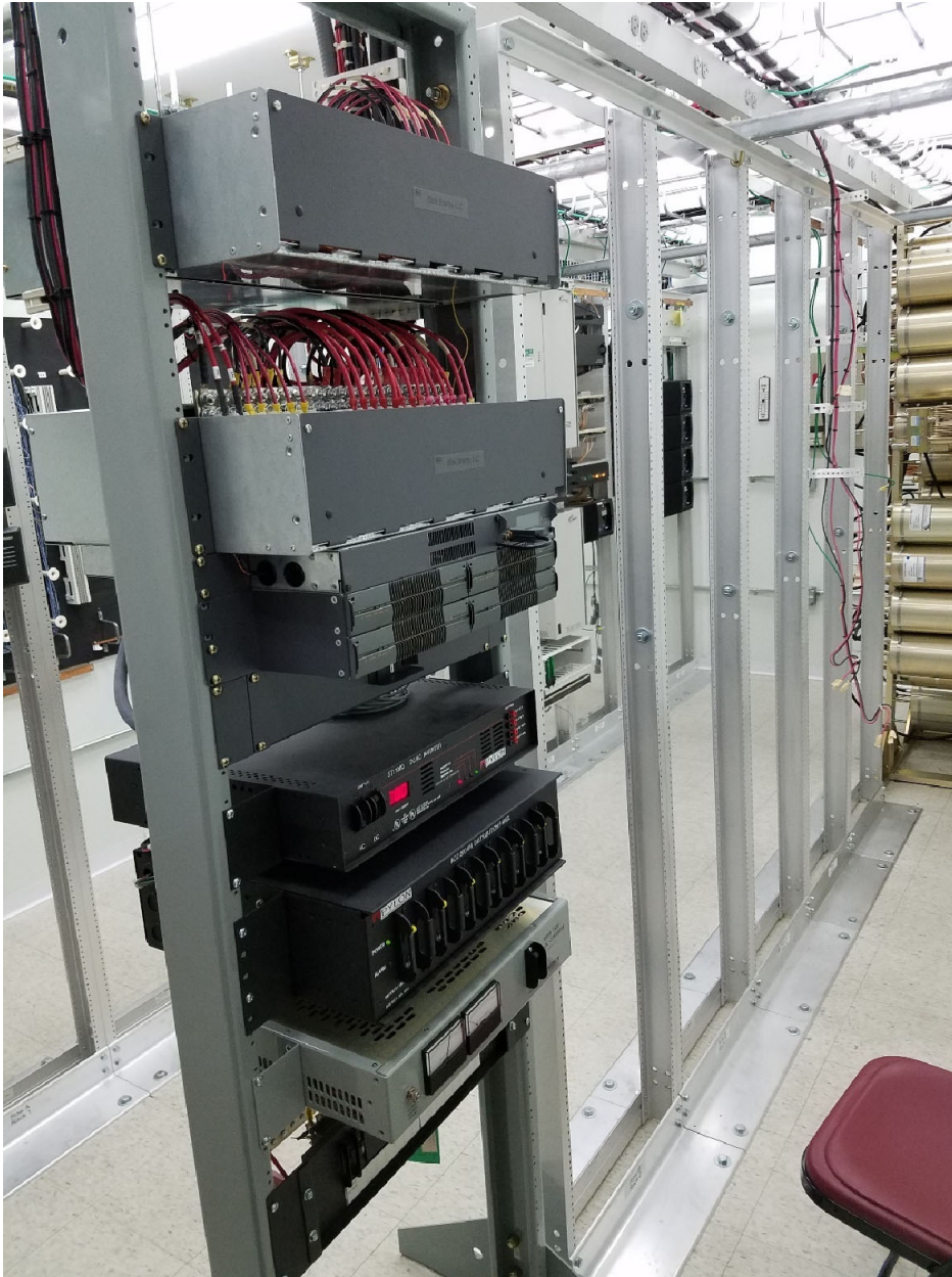
Figure 16: Orchard Heights DC Power Rack
