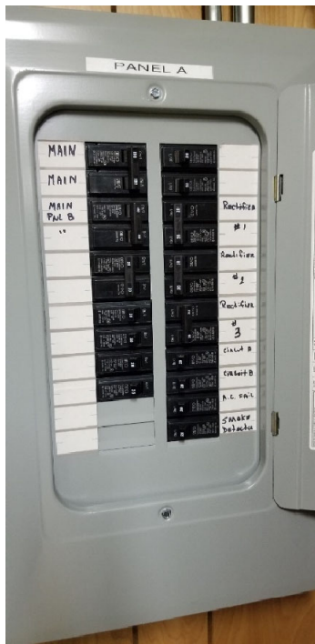
Figure 11: Lincoln Hill Main 120/240 VAC Panel (Note: 20A Rectifier Circuit Breakers)
