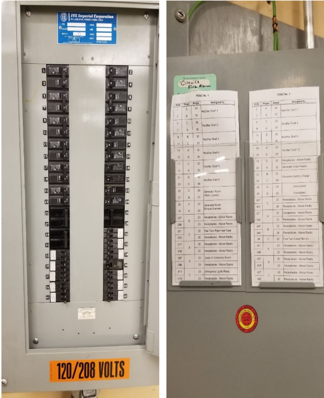
Figure 7: Gold Mountain 120/240 VAC Panel and Circuit Directory
