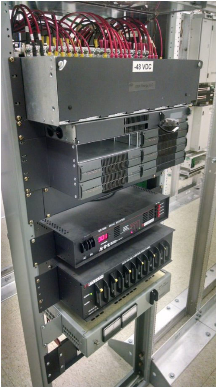
Figure 23: Suquamish DC Power Rack
