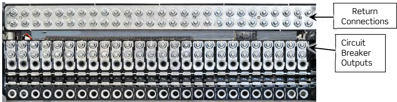
Figure 52 - Front Battery Connections (23" system shown)
