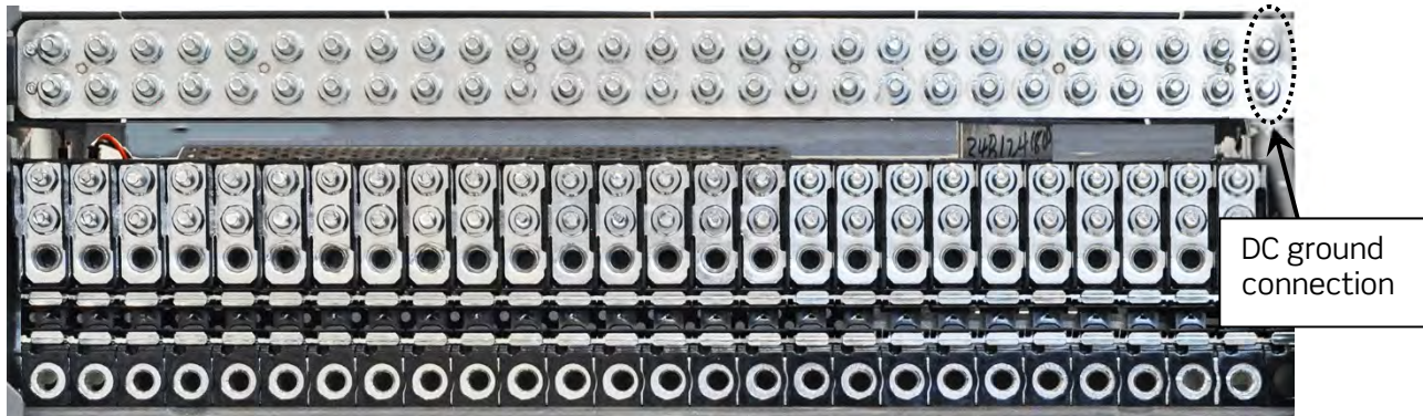
Figure 54 - DC Ground Connection, front
