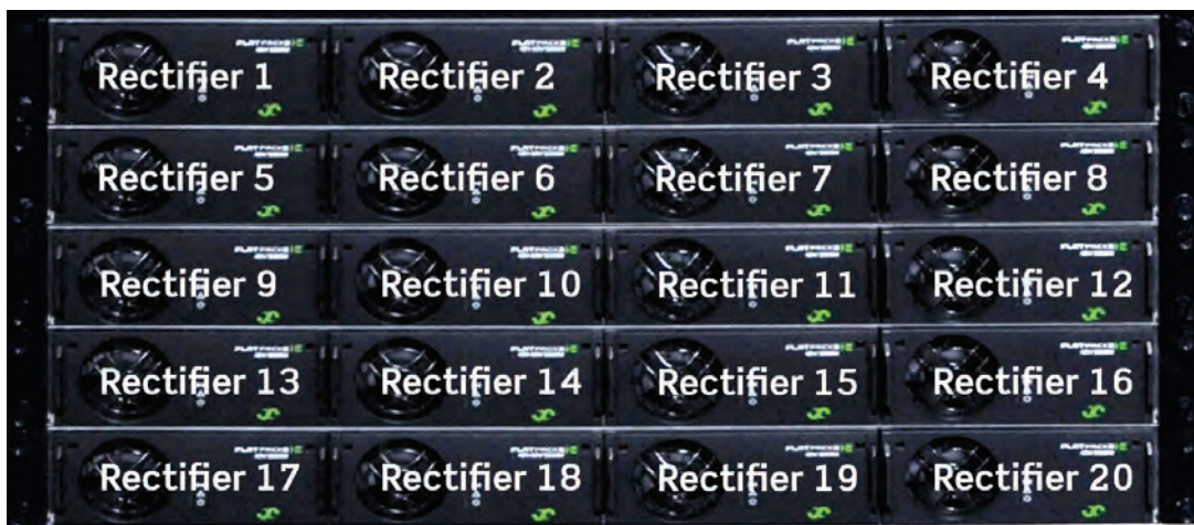
Figure 7 - Rectifier Slots (numerical order)
