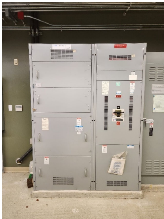
Figure 27: Photo 10 Utility Power Main Disconnect and Current Transformers (Front View)
