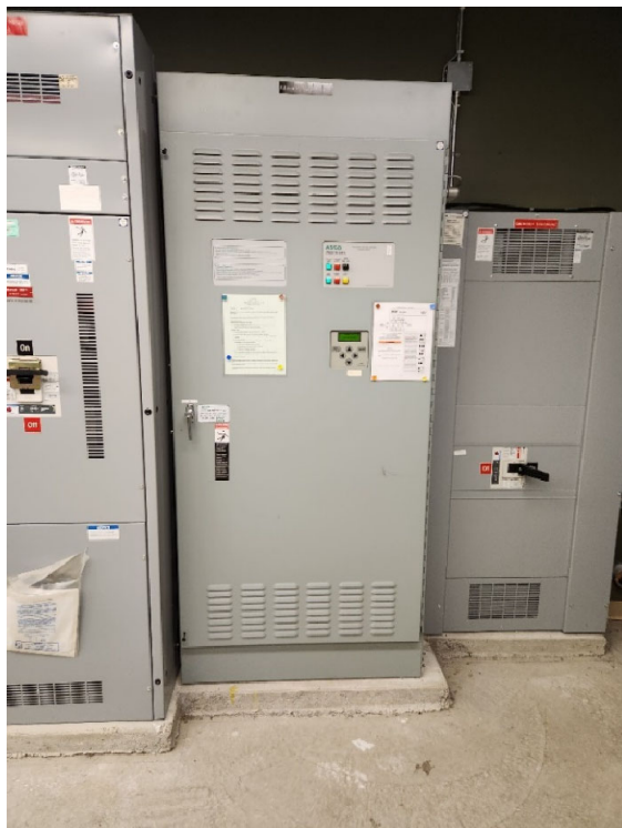
Figure 28: Photo 11 Automatic Transfer Switch and Generator Disconnect
