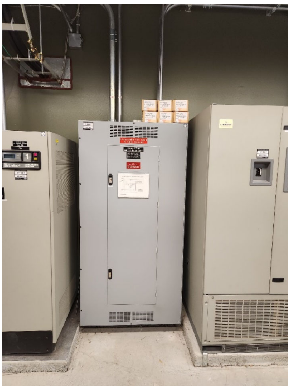
Figure 19: Photo 2 Maintenance Bypass Cabinet
