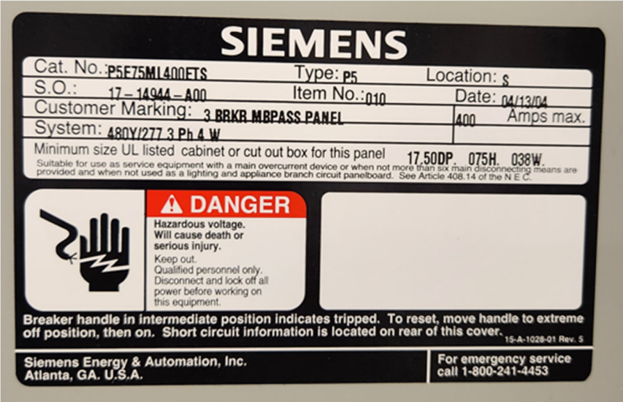
Figure 9: Maintenance Bypass Cabinet Nameplate
