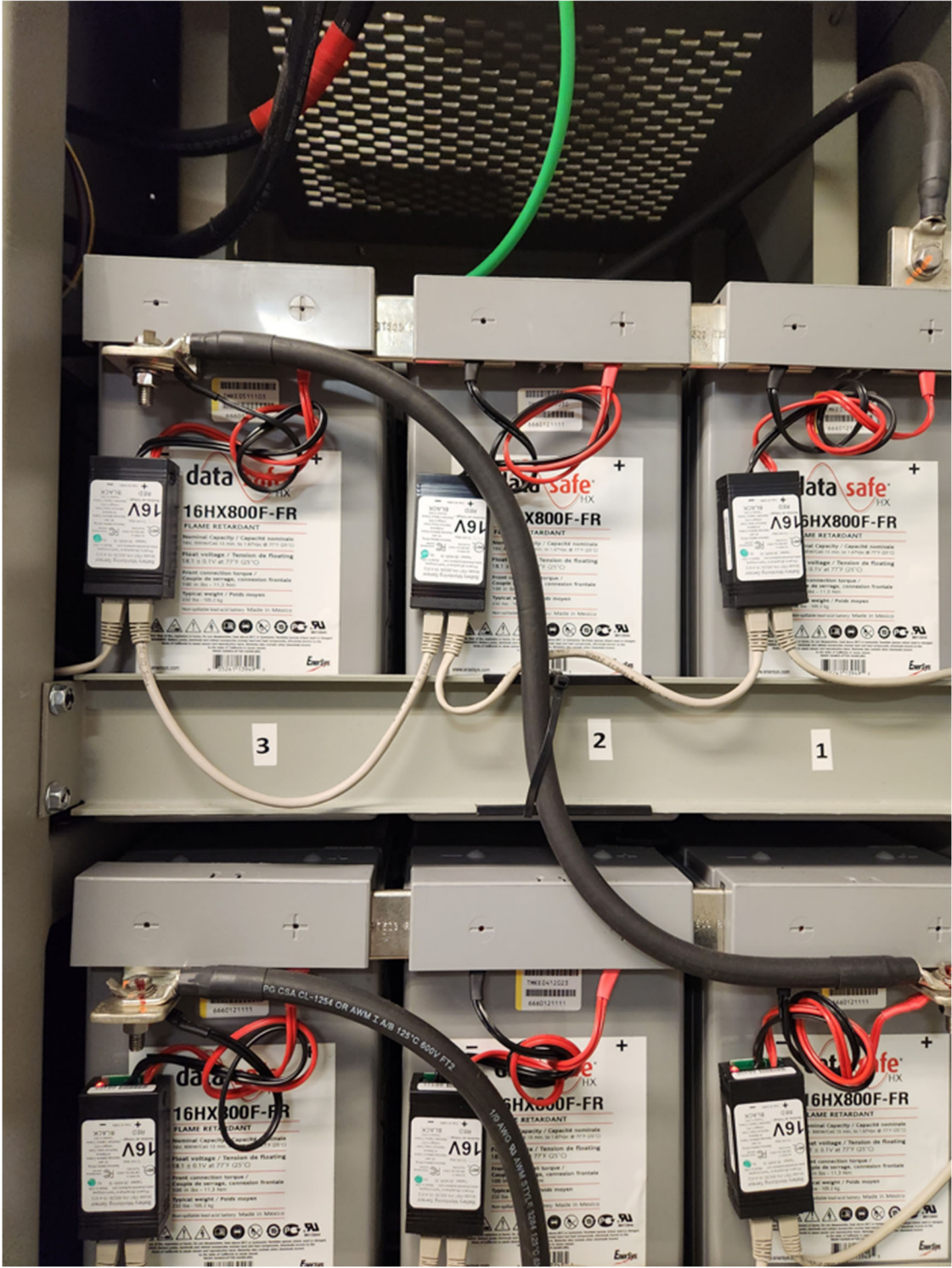
Figure 7: Battery Jars (2 strings, 30 jars each) Energys Data Safe 16HX800F-FR and Battery Monitoring System (Phoenix Broadband Technologies was acquired by SENS in March 2023)
