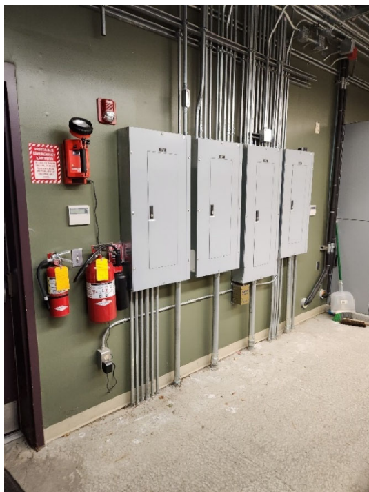
Figure 25: Photo 8 Electrical Distribution Panels
