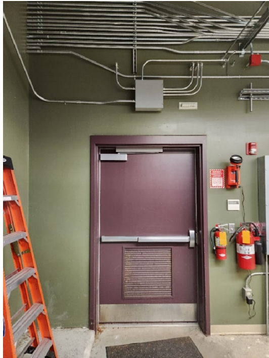
Figure 24: Photo 7 Exterior Electrical Room Door (48 inch to ground level, no curbs)
