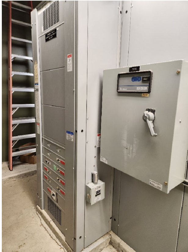
Figure 33: TVSS and 480V Distribution Cabinet
