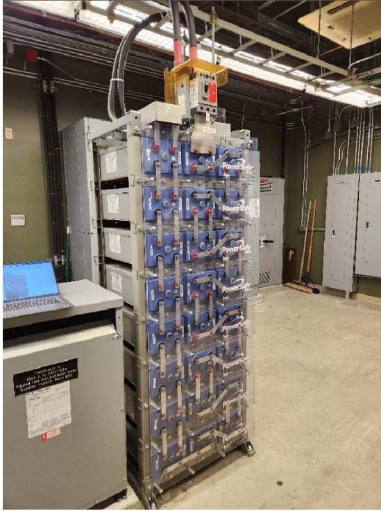
Figure 31: Transformer DB and DC Rectifier Batteries
