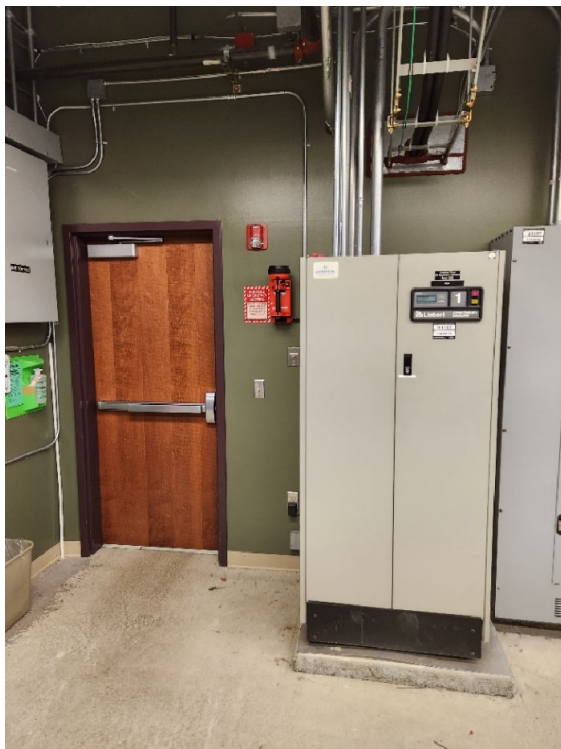
Figure 18: Photo 1 Electrical Room Interior Door and PDA
