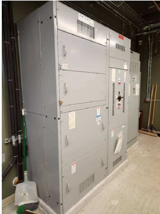
Figure 26: Photo 9 Utility Power Main Disconnect and Current Transformers
