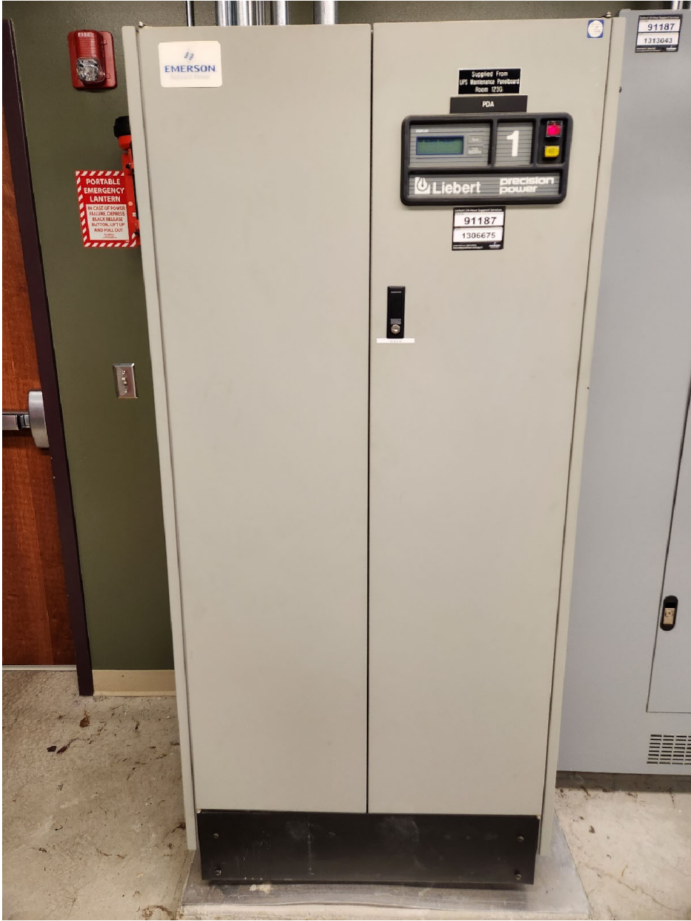
Figure 11: PDA – UPS Power Distribution Unit A
